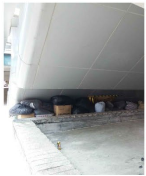
Existing Footbridge: Security and safety concerns
