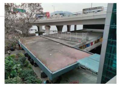
Top view of Kwun Tong Ferry Pier with Kwun Tong Bypass above
